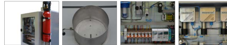
CO 2 fire suppression equipment
